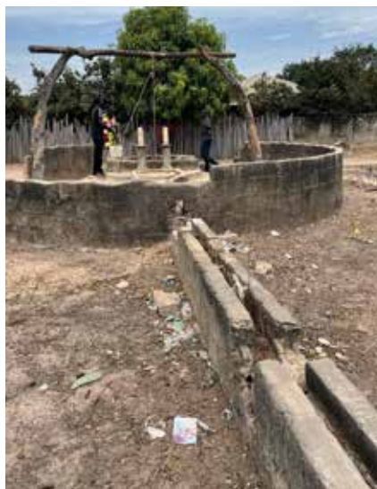
Broken lift pump.
